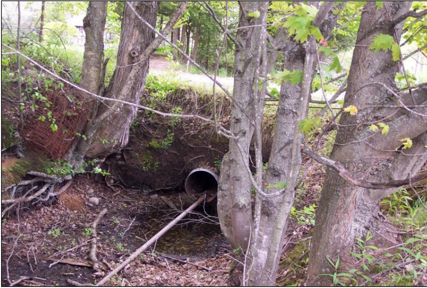
Before – Undersized culvert on the dry streambed
