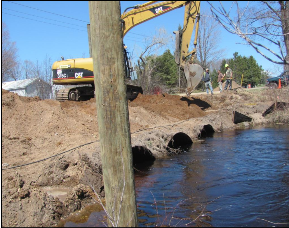
Emmet County Road Commission crew removing old culverts and old concrete footings and wing walls that were buried around the culverts from a previous crossing.
