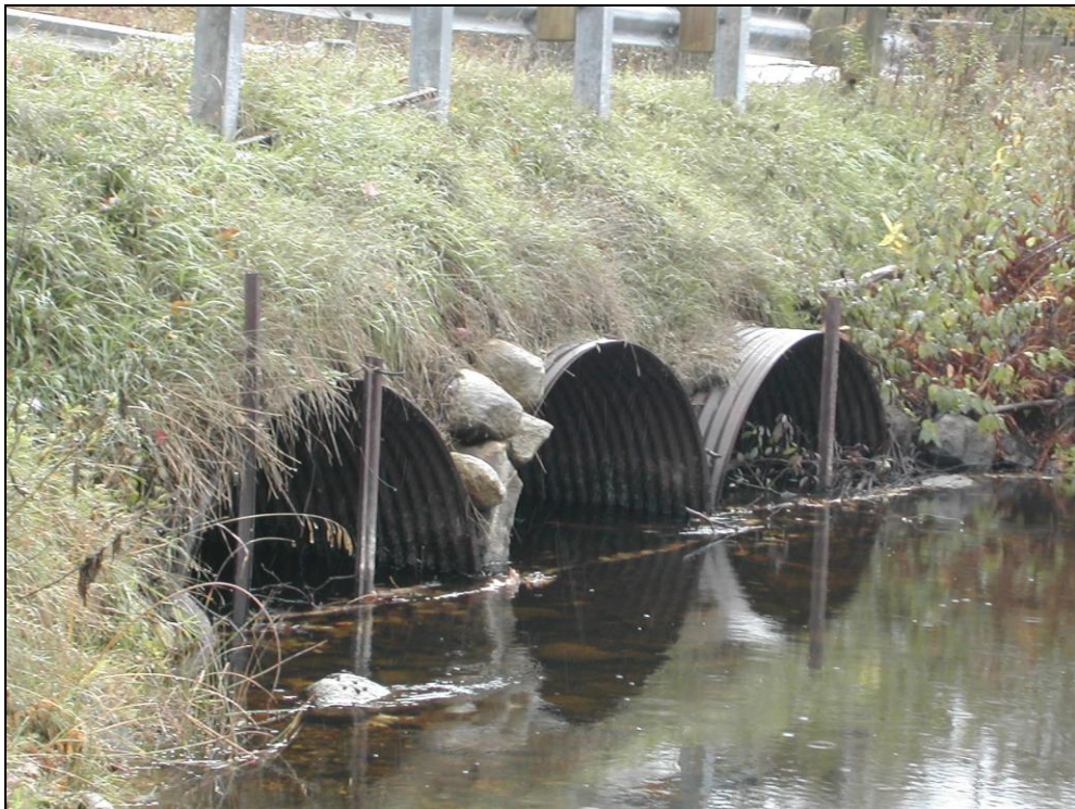
Close up of undersized failing culverts with attempts to keep debris from plugging tubes and creating flooding and failure potentials.
