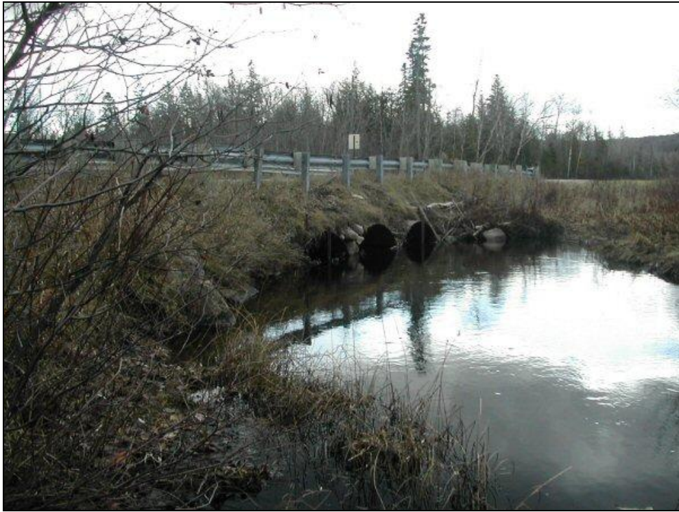
Failing culverts prior to construction. Culverts are severely undersized and incapable of handling stream flows. Pooling along the road is occurring. A 40' span timber bridge will allow for a natural stream channel and seasonal flows.
