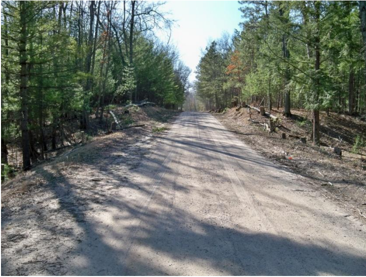
Steep approaches washed into stream – Before
