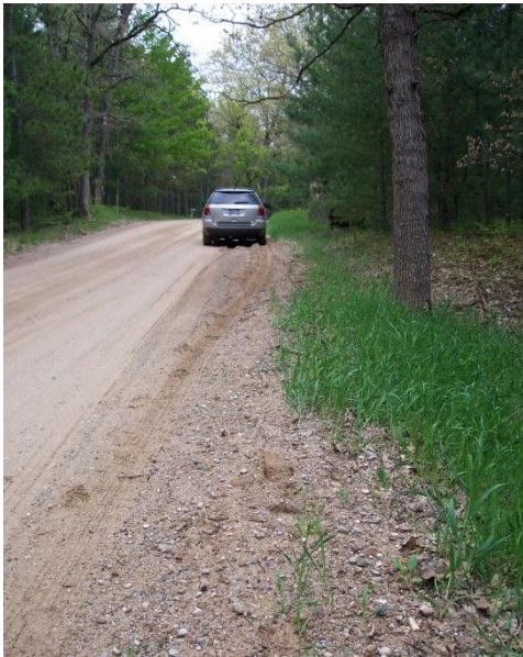
Eroding shoulders – Before
