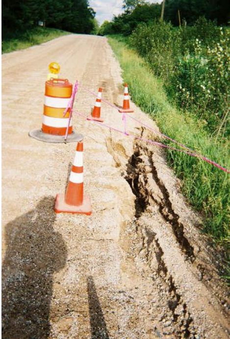
Severely eroding shoulders – Before
