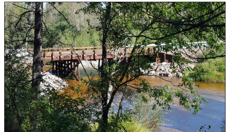
After - Guardrails and paving finished off the new bridge completed in September 2015
