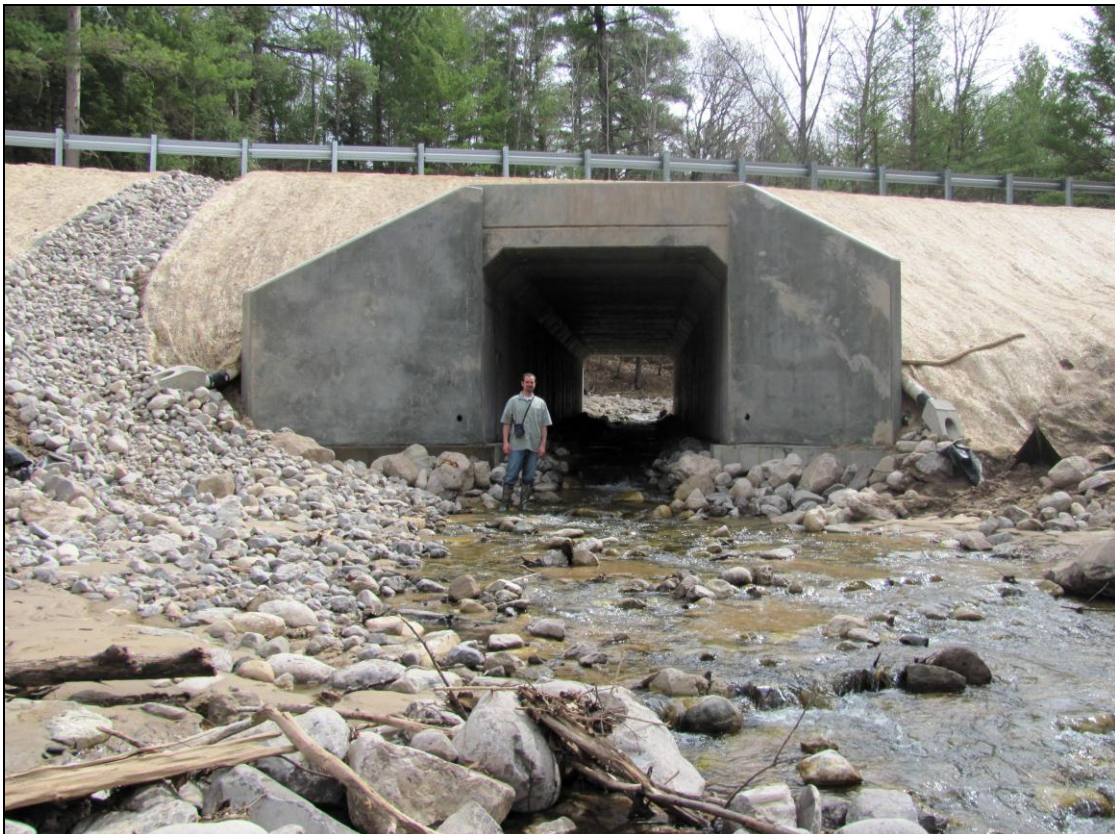
The completed structure includes paved approaches, runoff controls, and a clear span of the stream channel with virtually unlimited space for stream flow beneath the structure.
