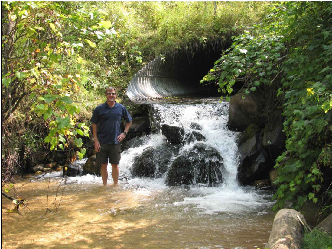
Perched culvert on Silver Creek completely blocking aquatic species passage approximately 400 yards from confluence with Pine River.
