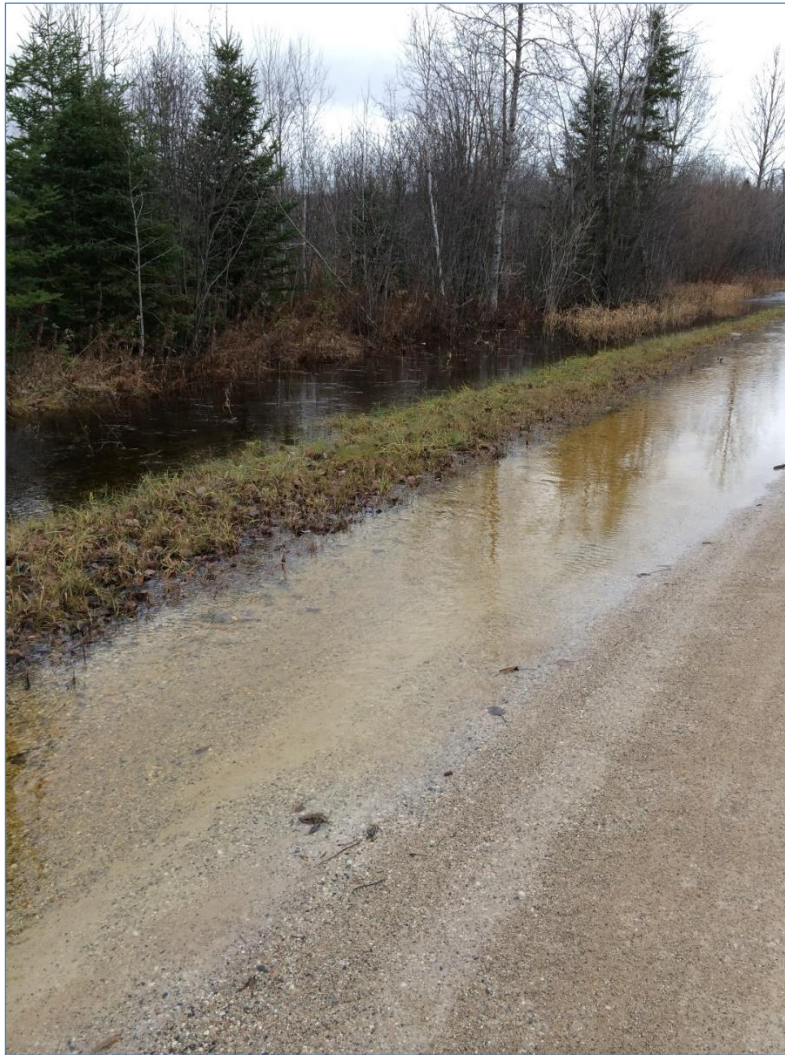
High waters often breached the culverts and road prism
